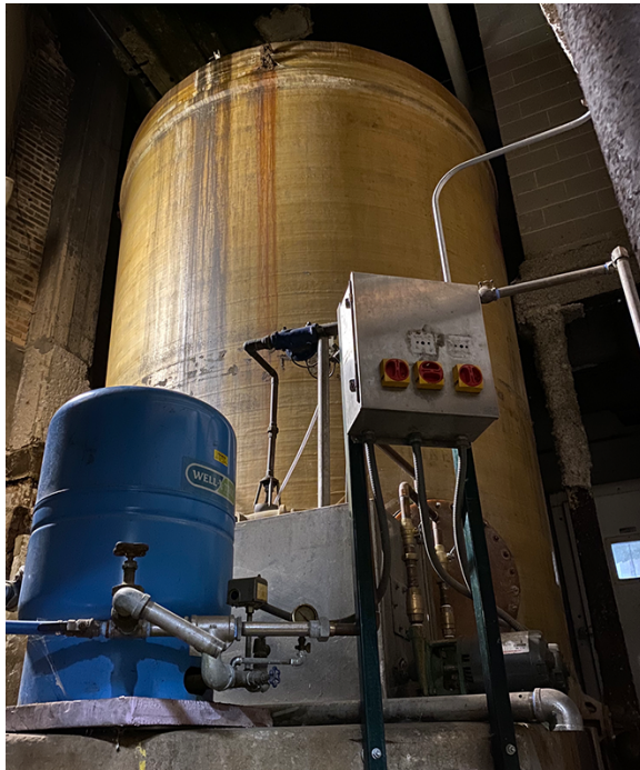
The brine tank, in background, with its break tank and connections to the water distribution system.
